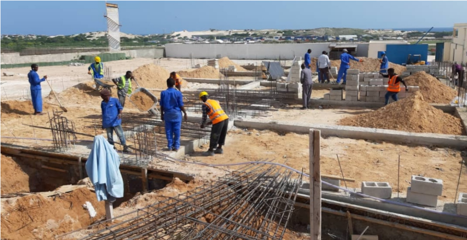
Construction work on the NIEC data centre and warehouse in progress and building is expected to be completed by the end of February 2020
